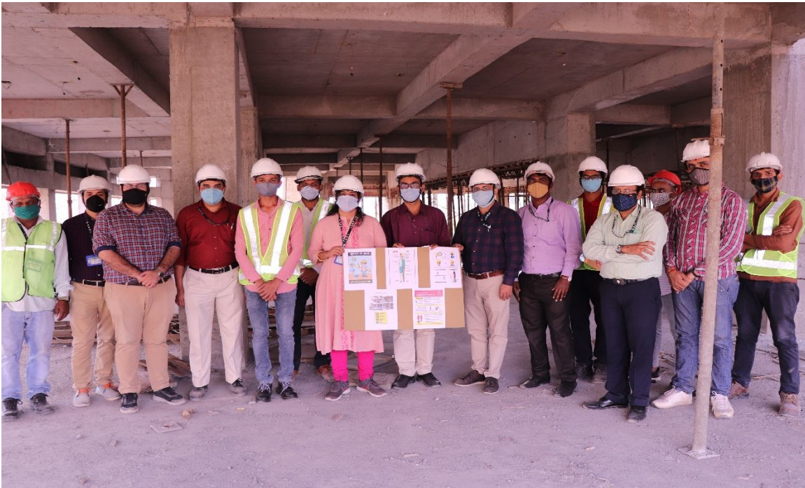
Visit by AERB Officials at construction site of Niyamak Bhavan-C to promote safety awareness among the construction workers on the occasion of National Safety Day-2021
